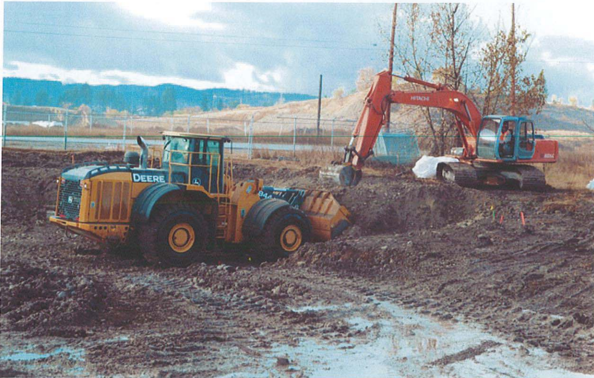
Photo 1: 11/2/10 - Loading soil from western side of lead-contaminated soils excavation at the KRY Site.
