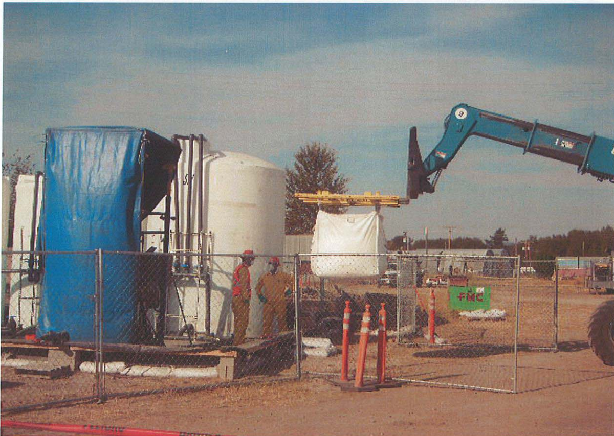
Photo 6: 9/14/11 - Super sack of dry persulfate being loaded into the mixer for use in chemical oxidation injections at the KRY Site.
