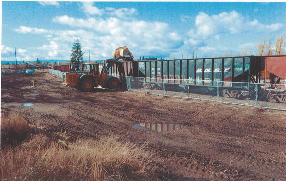
Photo 2: 11/2/10 - Loading lead-contaminated soils from the KRY Site into rail cars for transport to offsite disposal facility.
