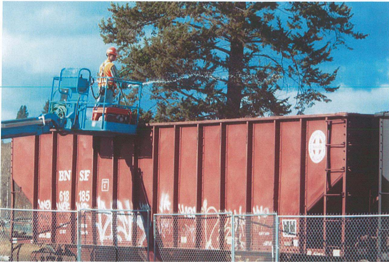
Photo 3: 11/2/10 - BNSF contractor spraying latex sealing compound to coat the top of the lead-contaminated soils in rail car to ensure contaminated soils don't blow out of rail car during transport to offsite disposal facility.
