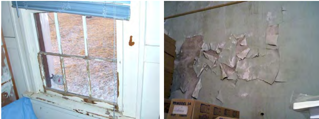
Left : Windows with failing wood frames and sashes. Right : Interior wall finish damage due to moisture penetration from the building exterior.
