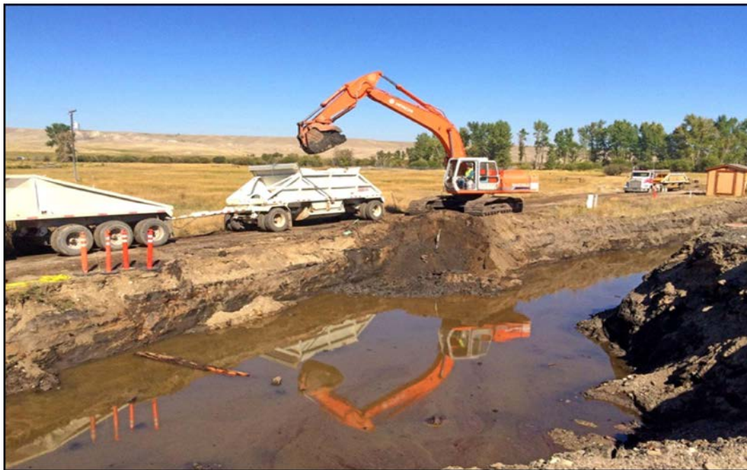
Excavating petroleum contamination at former Milwaukee Roundhouse facility in Deer Lodge (September 2015)
