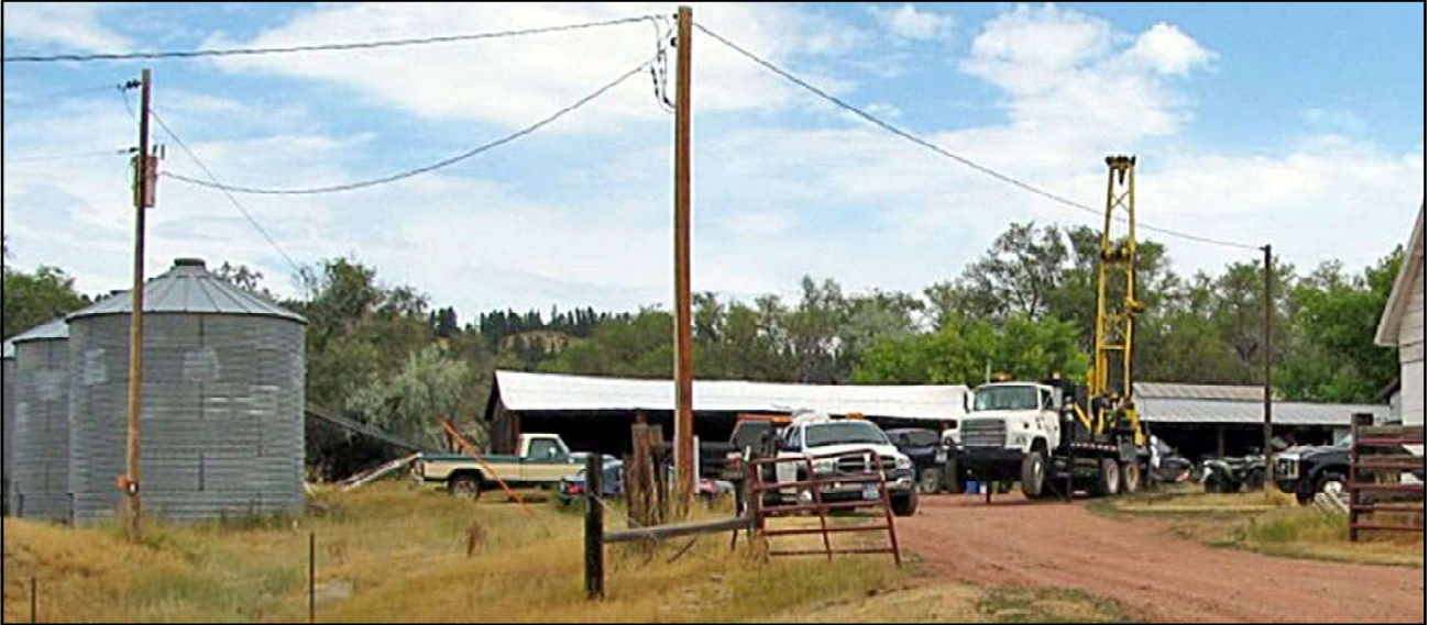
Drilling soil to verify cleanup of gasoline and diesel at rural farm near Decker (August 2016)
