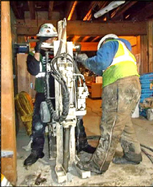
Drilling through basement floor to inject in-situ treatment chemicals near former dry cleaners, Havre (February 2016)
