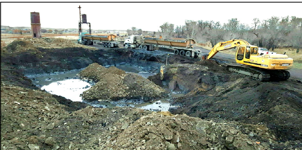
Excavating a leaking underground storage tank (LUST) and associated petroleum contaminated soil at former Chicago-Milwaukee Rail Yard, Harlowton (November 2016)
