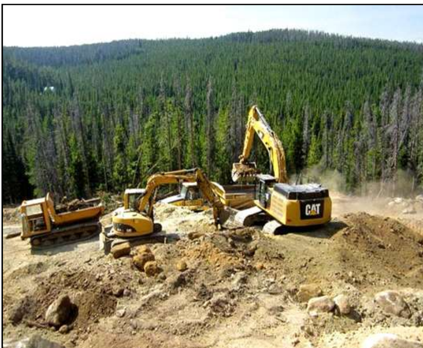
Removing mine tailings from abandoned mine in the headwaters of the Little Blackfoot River near Elliston (August 2016)
