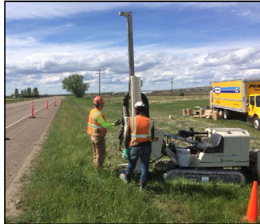
Injecting in-situ remediation chemicals to target petroleum migrating underneath Highway 2, Harlem (May 2017)
